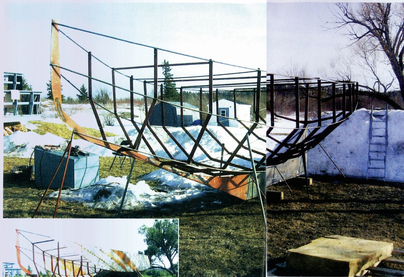
ABOVE Hull shape is established once keel, frames and chine are in place
